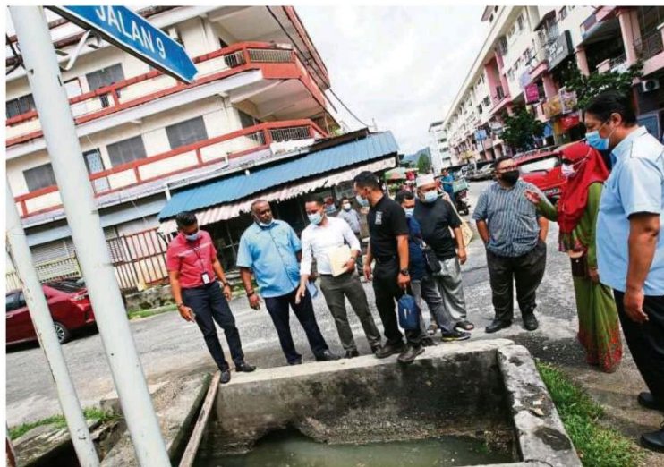
Deveandran (second from left) discussing with MPS officers and traders on the drainage rectification works needed to overcome flash floods at Selayang Centre Point in Selayang Baru.
